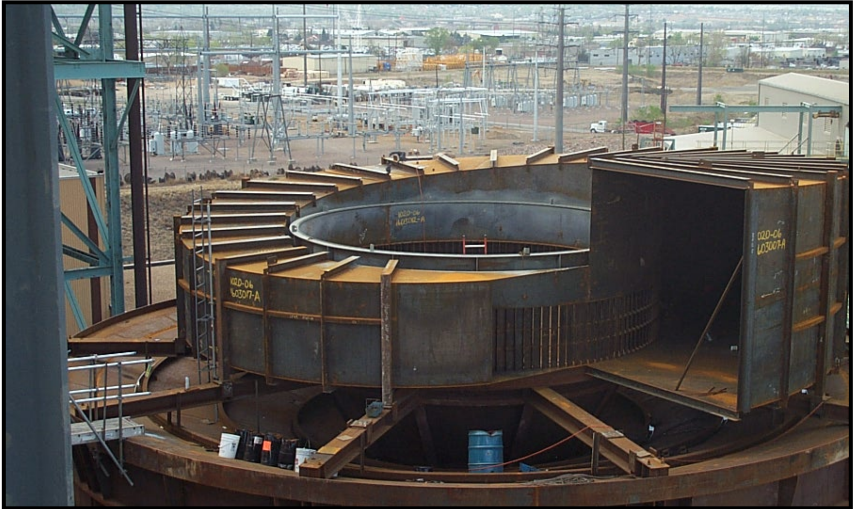
Roof Gas Disperser
